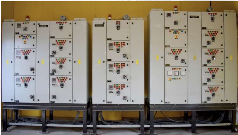
STARTER CUM CONTROL PANELS
