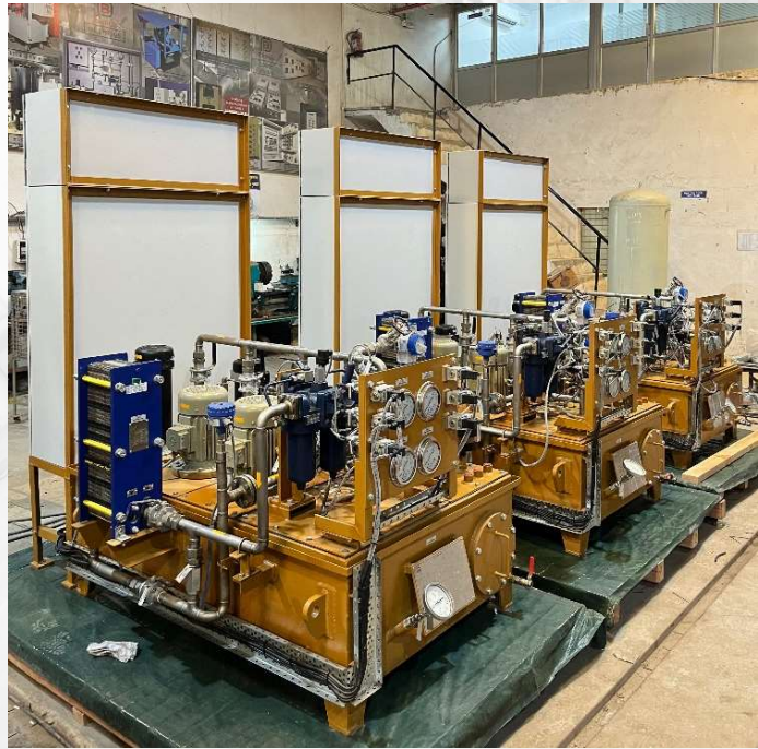
GENERATOR LUBRICATION OIL PLANT
